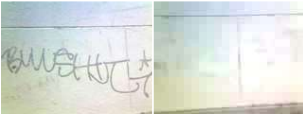
September 15, 2011: Corner of Castro & 18 th St. St. Graffiti Removed
