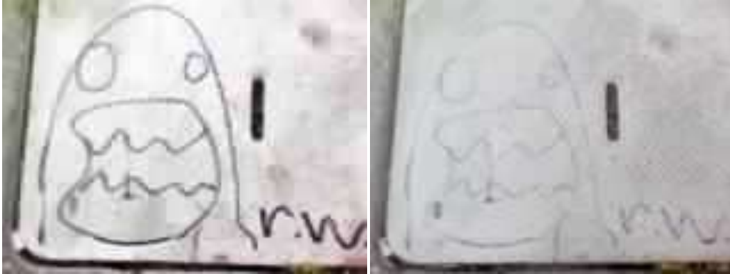
September 22, 2011: 2095 Market St. Graffiti Removed, Repaint needed
