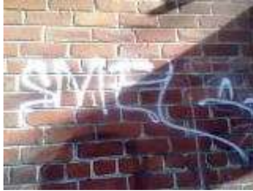
October 8, 2011: 1903 Market St. Will need power washing
