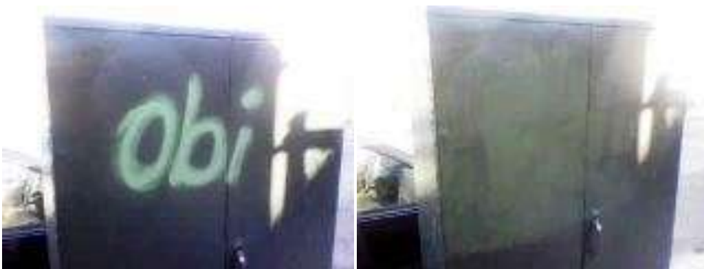
October 21, 2011: 133 Elgin Park, Graffiti Removed
