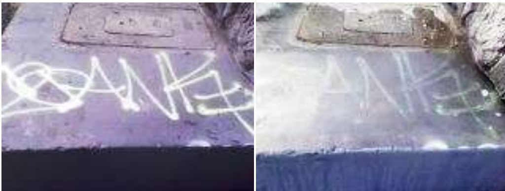
May 29, 2011: 1946 Market St. Removal attempted, steam clean needed
