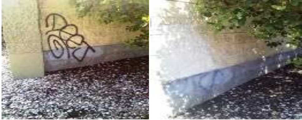
May 20, 2011: Safeway area- Church St. Graffiti Removed
