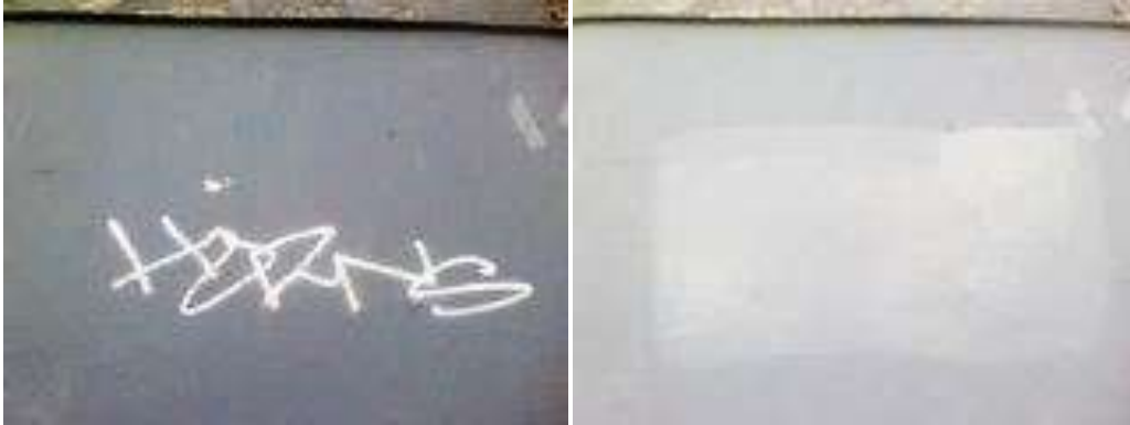
June 24, 2011: 1874 Market St. Graffiti Removed
