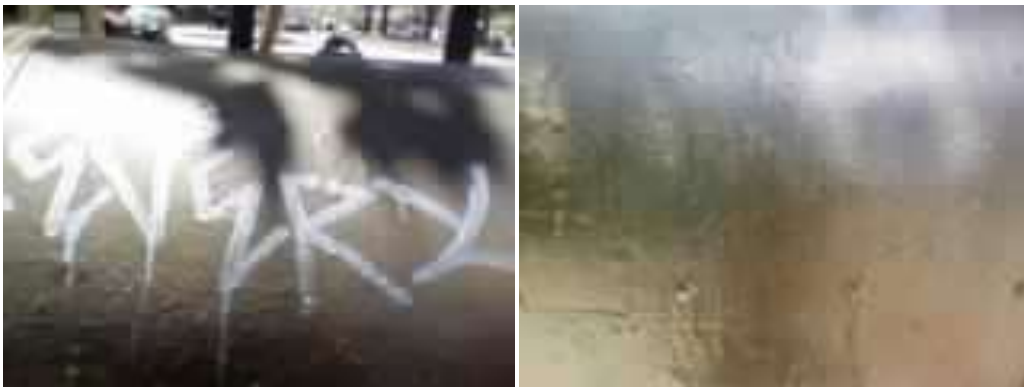
June 2, 2011: 1939 Market St. Graffiti Removed
