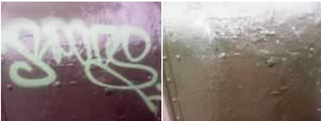
June 29, 2011: 1817 Market St. Graffiti Removed
