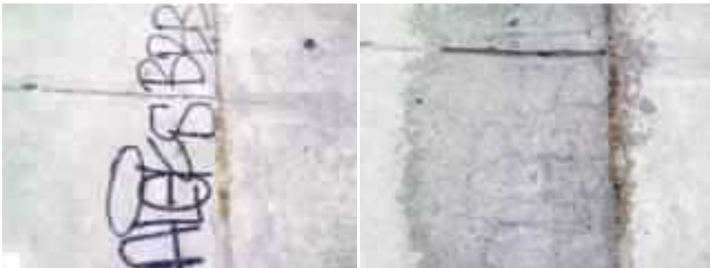
June 27, 2011: 2200 Market St. Graffiti Removed
