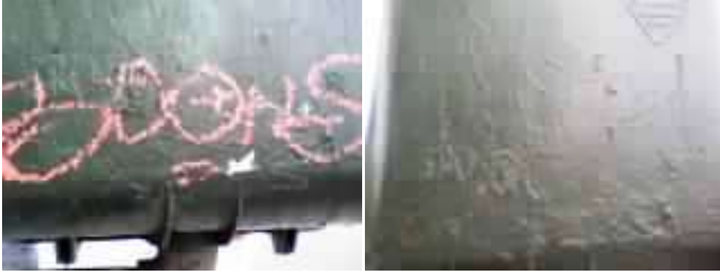
June 3, 2011: 2189 Market St. Graffiti Removed
