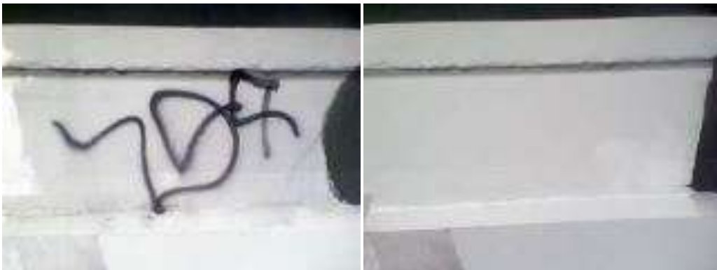
June 12, 2011: 133 Elgin Park, graffiti removed
