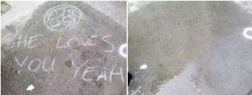
June 27, 2011: 2073 Market St. Graffiti Removed
