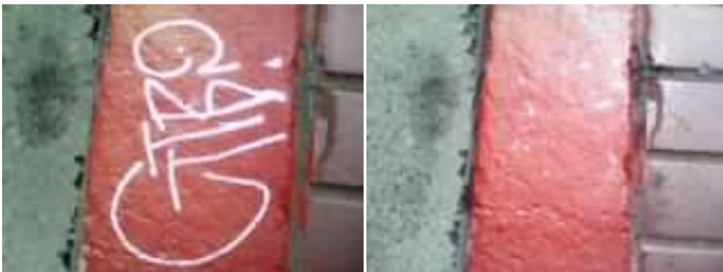
June 1, 2011: 1946 Market St. Graffiti Removed
