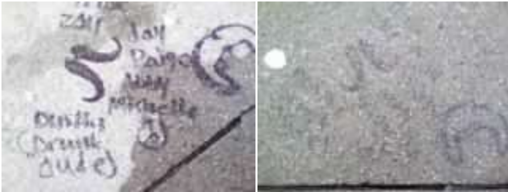
June 27, 2011: 411 Castro St. Graffiti Removed
