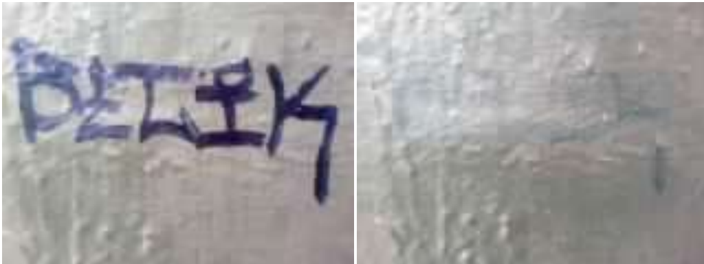
June 29, 2011: 1975 Market St. Graffiti Removed
