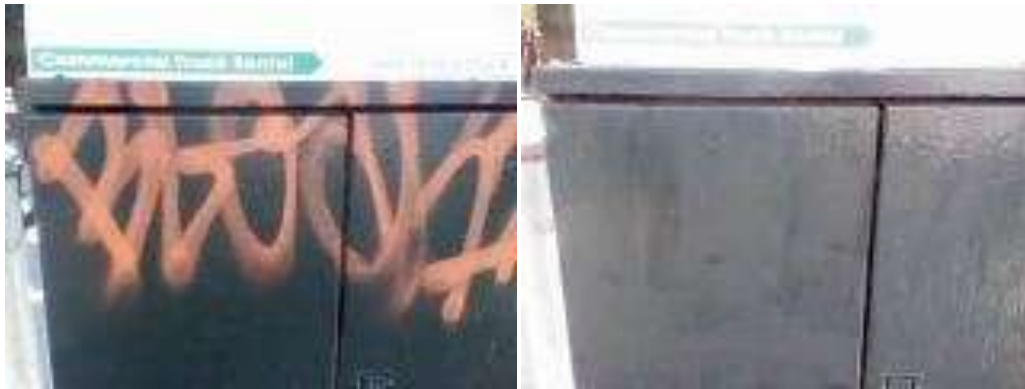
Sample of Graffiti Removed
