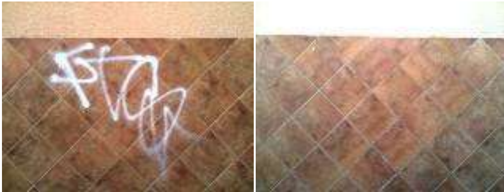
April 26, 2011: 4201 18 th St. Graffiti Removed
