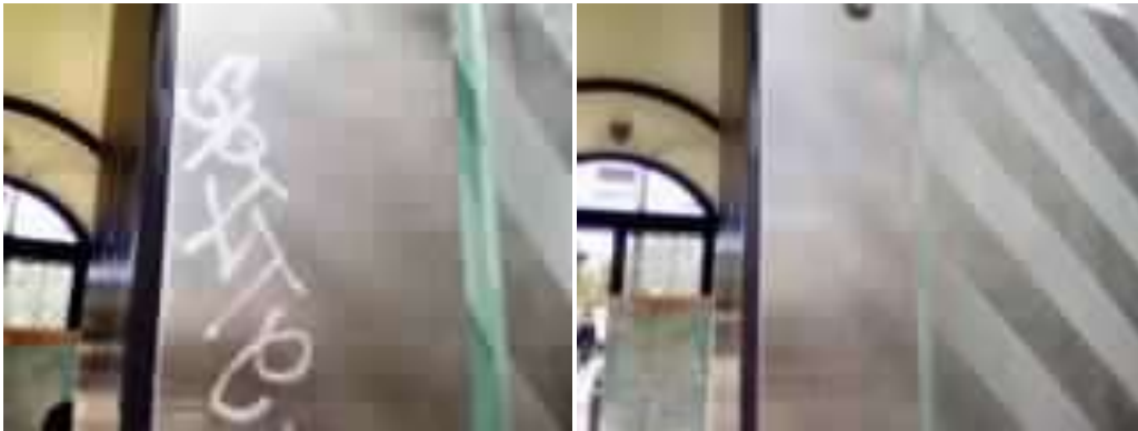
April 9, 2011: 3985 17 th St. Graffiti Removed
