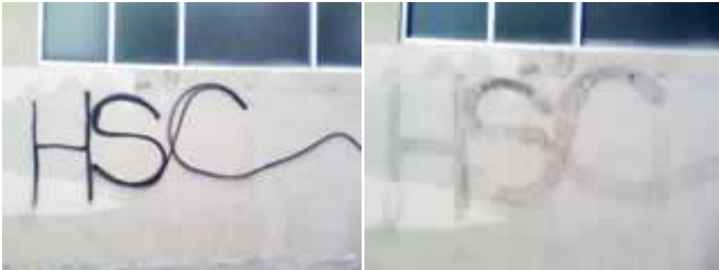
April 14, 2011: 2001 Dolores St. Graffiti Removed, Repaint needed
